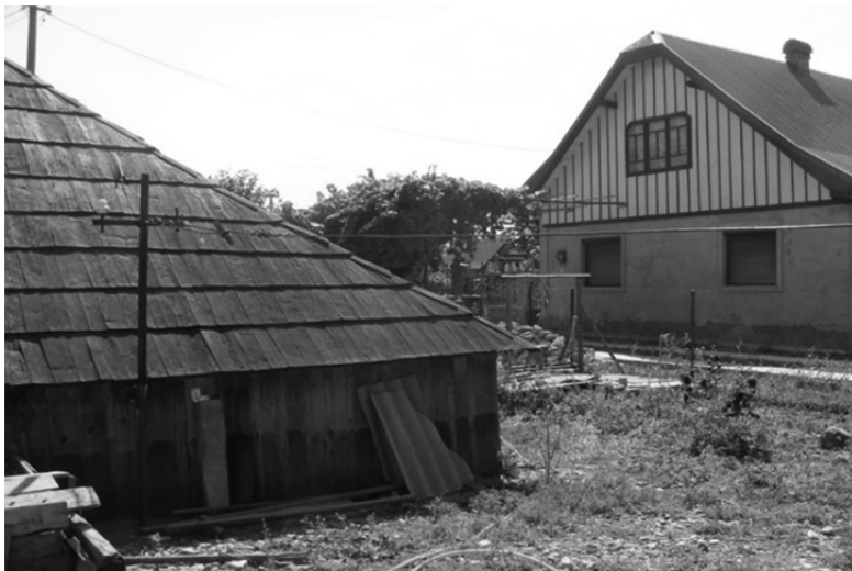
Figure 8. The northern slope of the roof goes down unto the ground (Author personal photo).
