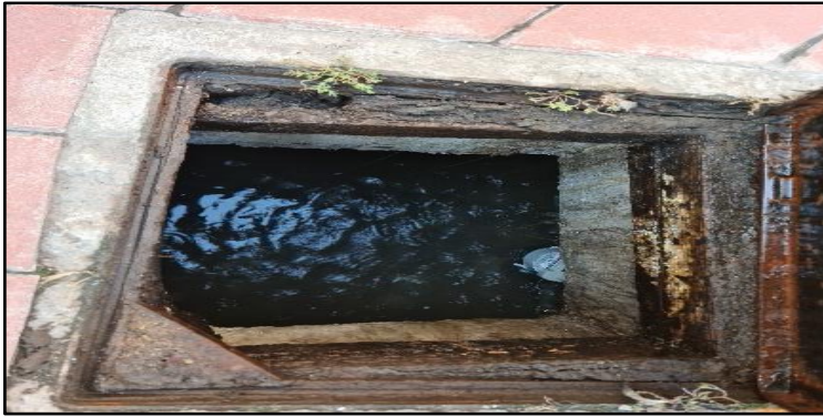
Fig. 8. Outdoor main building water pipe rupture Source: Author's personal household
